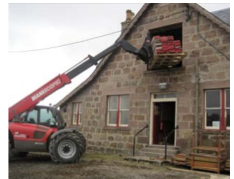
^ Work being carried out to the hall, including increased wall insulation and new timber partitions.
