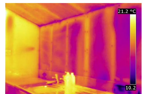
Thermographic images in the kitchen from April 2012 (top) and March 2014 (bottom) illustrating the positive effect of increased insulation
