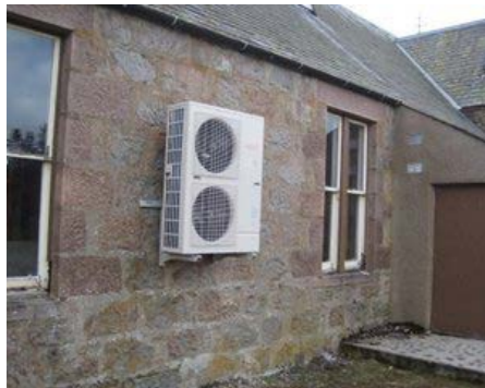
Air source heat pump
