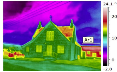
Thermographic images of the exterior from April 2012 (top) and March 2014 (bottom) illustrating how increased insulation has eradicated cold spots at the eaves, around the windows and at the corners of the building. Heat Loss from the unimproved small hall is very evident.
